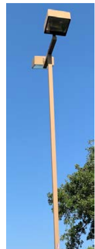
Figure 1 - Older HID Shoebox Fixture
